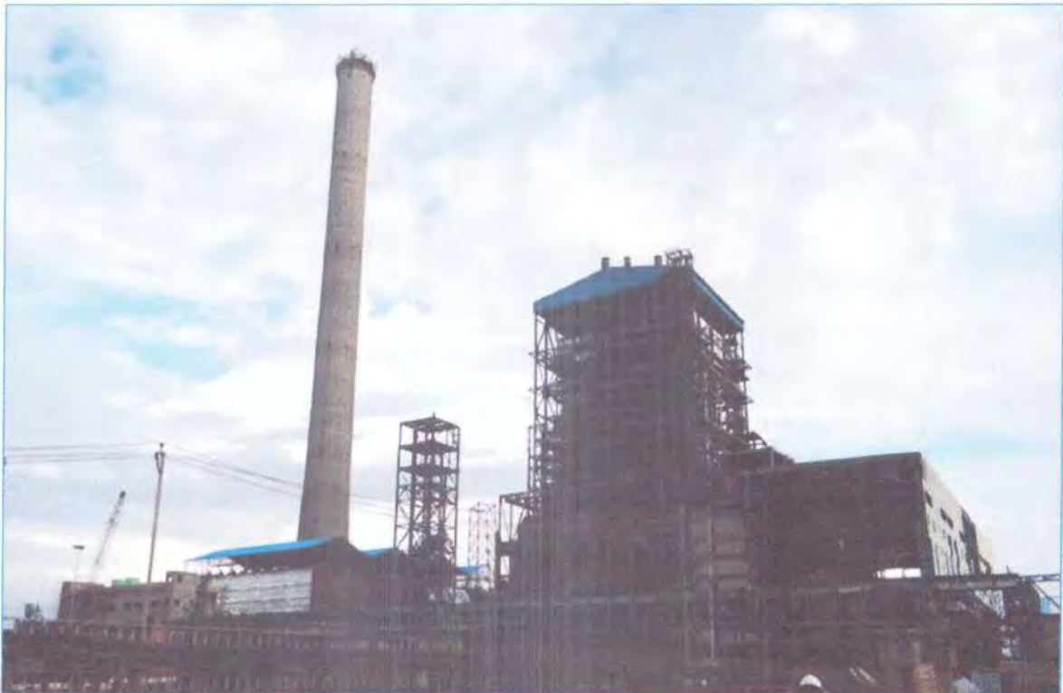
Figure No.1. Raigarh Energy Generation Ltd.
