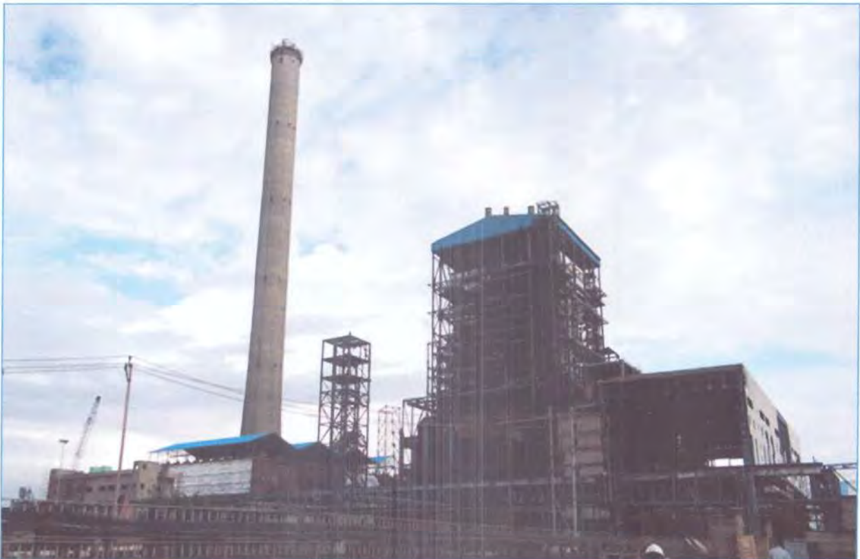
Figure No.1. Raigarh Energy Generation Ltd.
